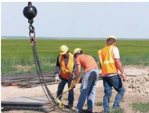
Construction workers prepare the site for the Judith Gap Wind Farm. PHOTO: Windpark Solutions America
