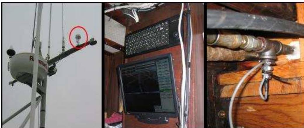
Figure 3. Examples of sensor installations on the study vessels: GPS receiver (left), monitor and keyboard (center), and hydraulic pressure sensor (right).
