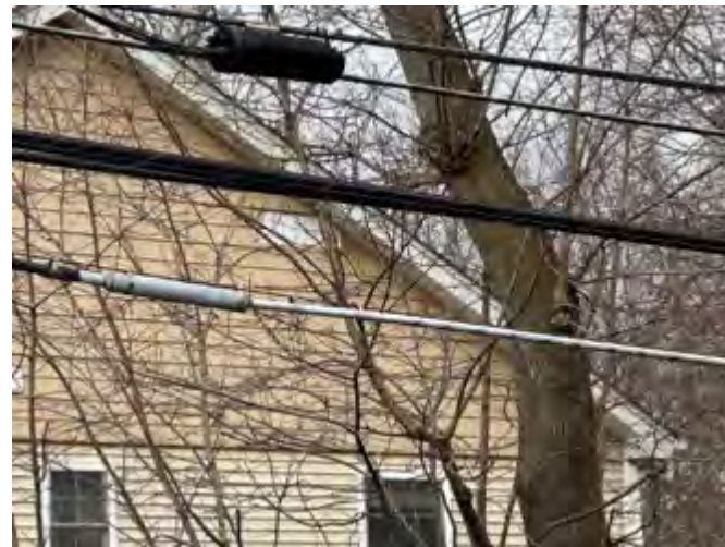
(C) Exposed bare lead splice box and lead cable. January 2023. Highland Falls, New York.
