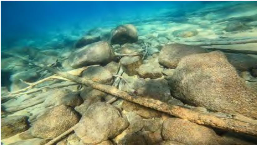
(D) Lead sheathed cable laying among boulders on the lake bottom. April/March 2022. Lake Tahoe, California.
