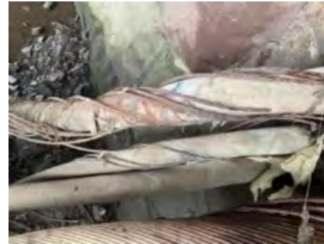
(K) Close up of cables at Passaic 8. January 2023. New Jersey.
