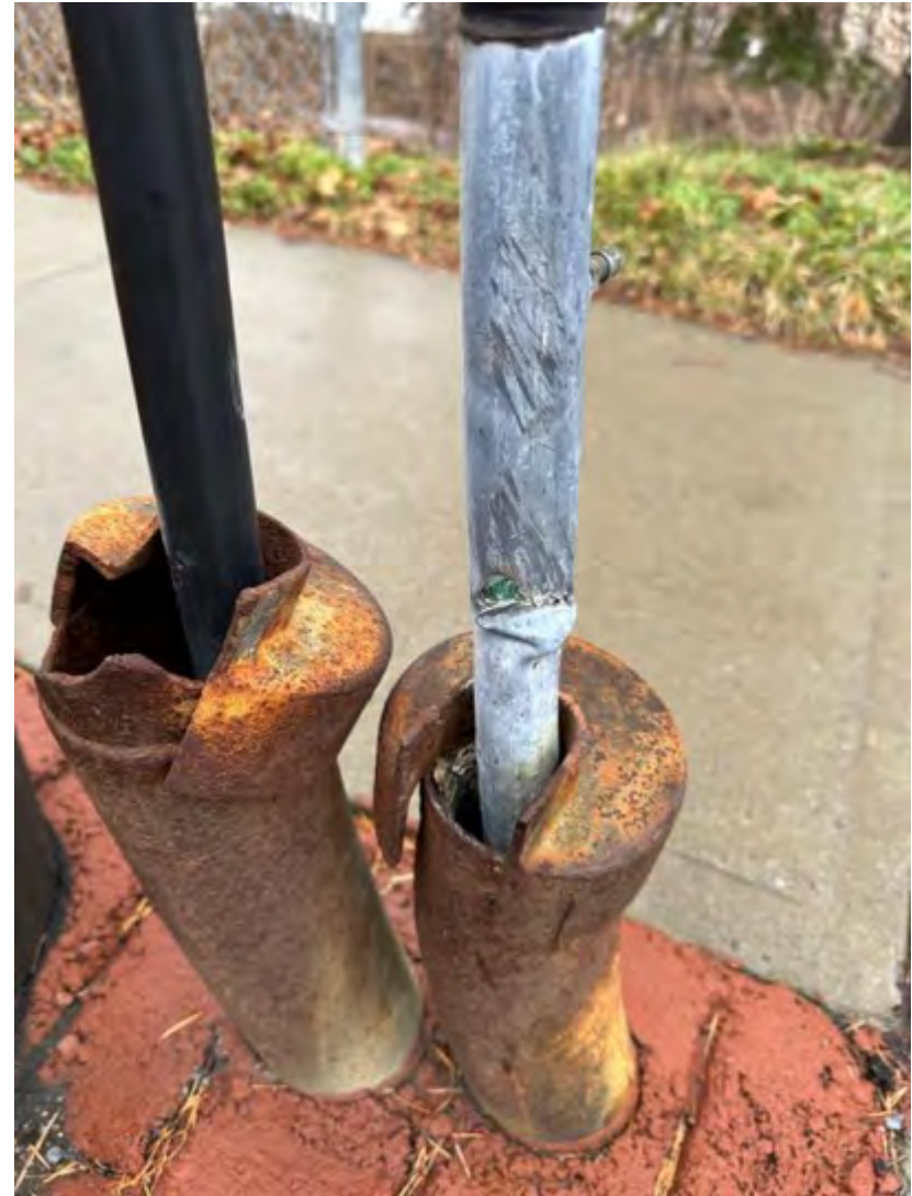
(L) Close up of damaged lead sheathed cable shown in (K). Wappingers Falls 3. January 2023, Wappingers Falls, New York.
