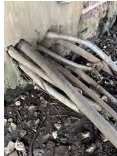
(L) Part of an eleven-cable location found near Wall Street Bridge, between Garfield and Wallington. Passaic 8. January 2023. New Jersey.
