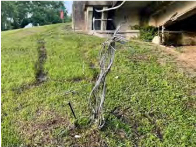
(C) Remnants of bare lead sheathed cable and steel wire below the Bridge Street Bridge. BT 1.1. June 2022, New Iberia, Louisiana.
