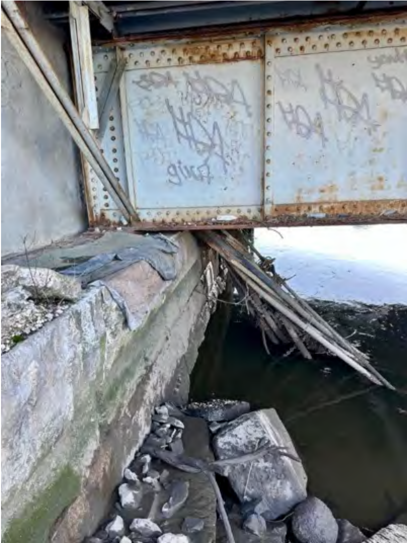
(H) Evidence of homeless sleeping next to these cables along the Passaic River. Passaic 2. January 2023, Harrison/University Heights, New Jersey.
