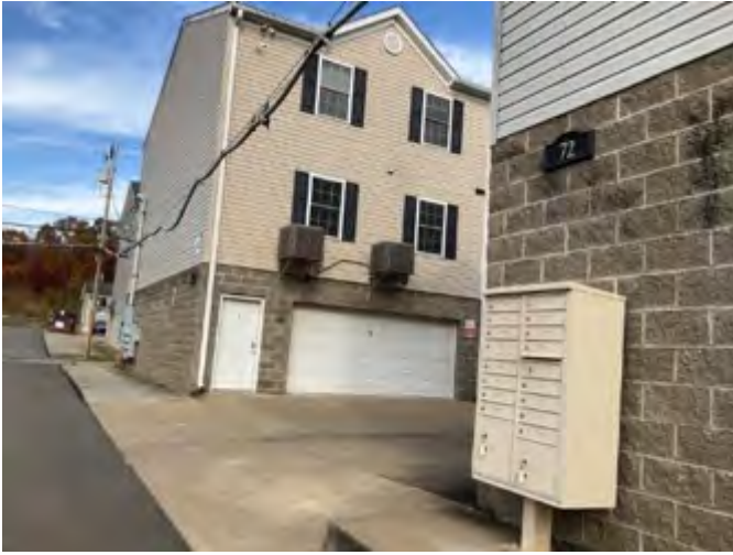
(D) CT6. Overhead lead sheathed cable running across the entrance into apartments and over access to mailboxes. February 2023. Coal Center, Pennsylvania.
