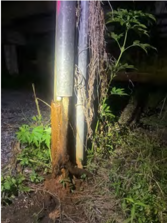
(B) Old telephone pole with cable guard and old conduit where a cable would have been. There is currently corrugated plastic hose behind the guard and in the steel pipe, but no visible cable. BL 2.2. Labadieville, Louisiana. June 2022.
