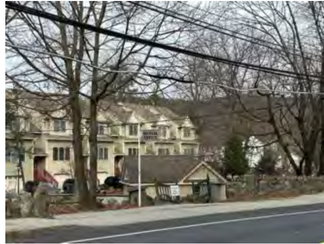
(B) Overhead lead sheathed cables in front of an apartment complex. January 2023. Highland Falls, New York.
