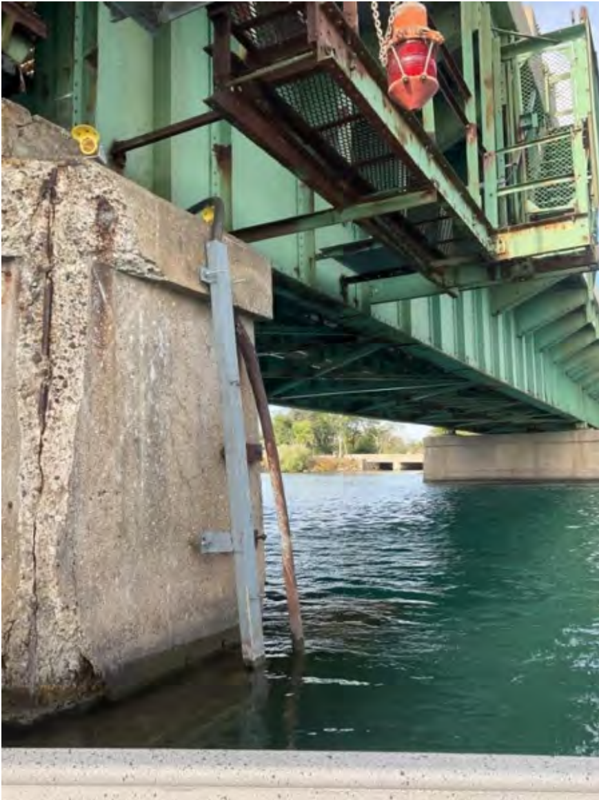
(E) Lead sheathed cable along the Grosse Ile Parkway Bridge. The cable runs through the concrete and is cut just above the ledge. DR 2. Grosse Ile Township, MI
