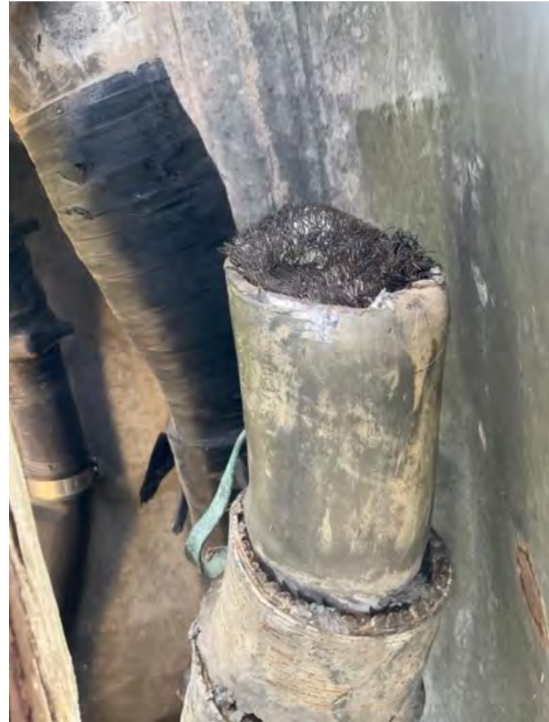
(N) Donaldsonville, LA. Location MISS 12.1. Close up of lead sheathed cable next to lead splice box seen in (K). June 2022.
