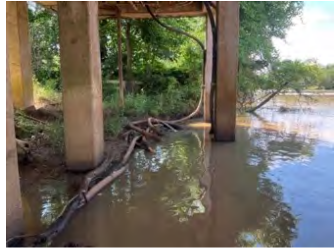
(E) Rd. 320 southeast of New Iberia, LA. Cluster of lead sheathed cables under the Oliver Bridge. BT 17.1. June 2022, New Iberia, Louisiana.
