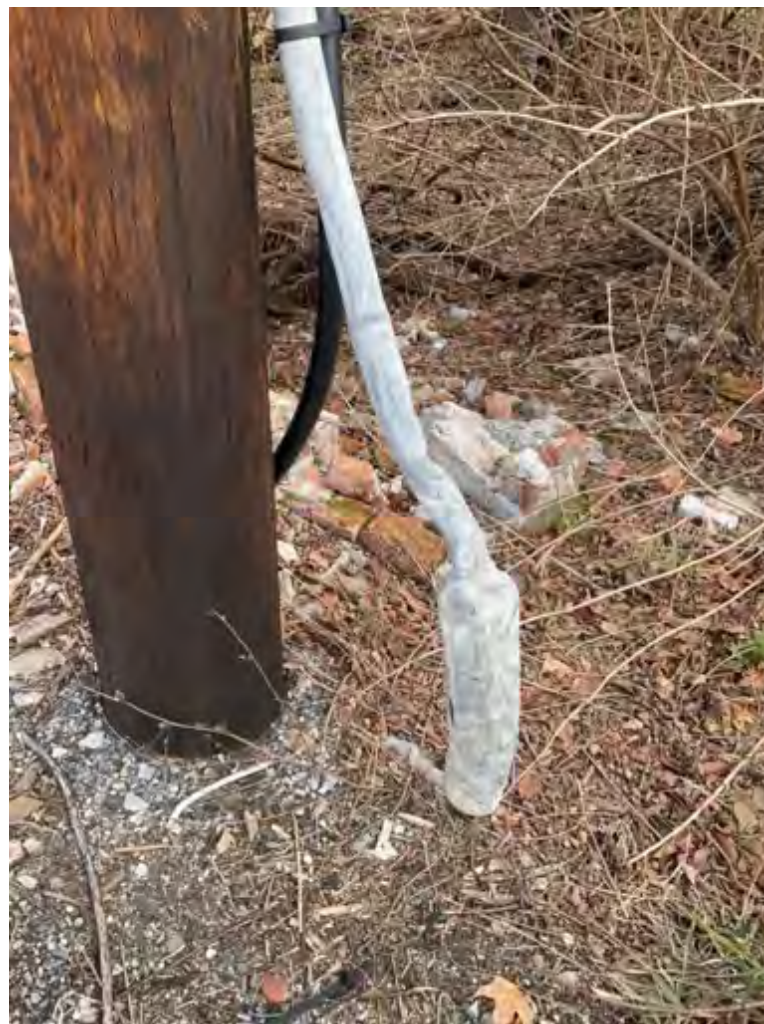
(G) Damaged lead cable and splice box at the base of an old telephone pole. Point of Interest: New Windsor 1. January 2023, New Windsor, New York.
