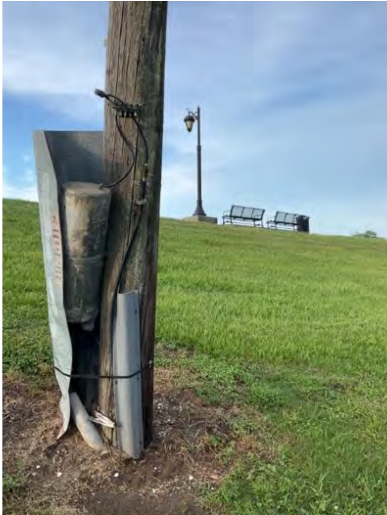
(M) Donaldsonville, LA. Location MISS 12.1. Exposed leaded splice box that appears to still be connected to an air test line. See photo (L) for the abandoned cable just the other side of the splice box. June 2022,
