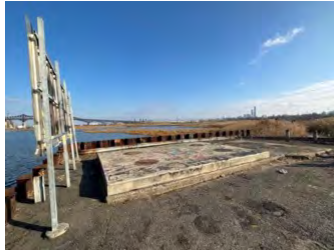
(C) Vault area looking towards Lincoln Park Wetlands & Nature Trail. January 2023, West Side, New Jersey.
