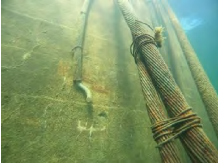
(E) Close up of small, cut, bare lead sheathed cable underwater. Site LP 4.1. August 2022, Lake Pend Oreille, ID.
