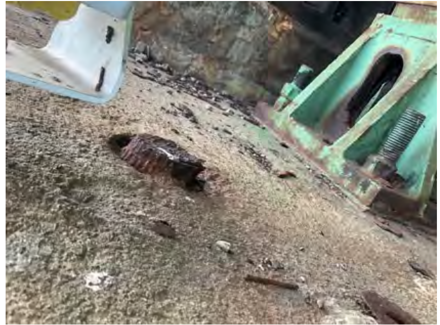
(F) Cut lead sheathed cable, referenced in (E). DR 2. Grosse Ile Township, MI.
