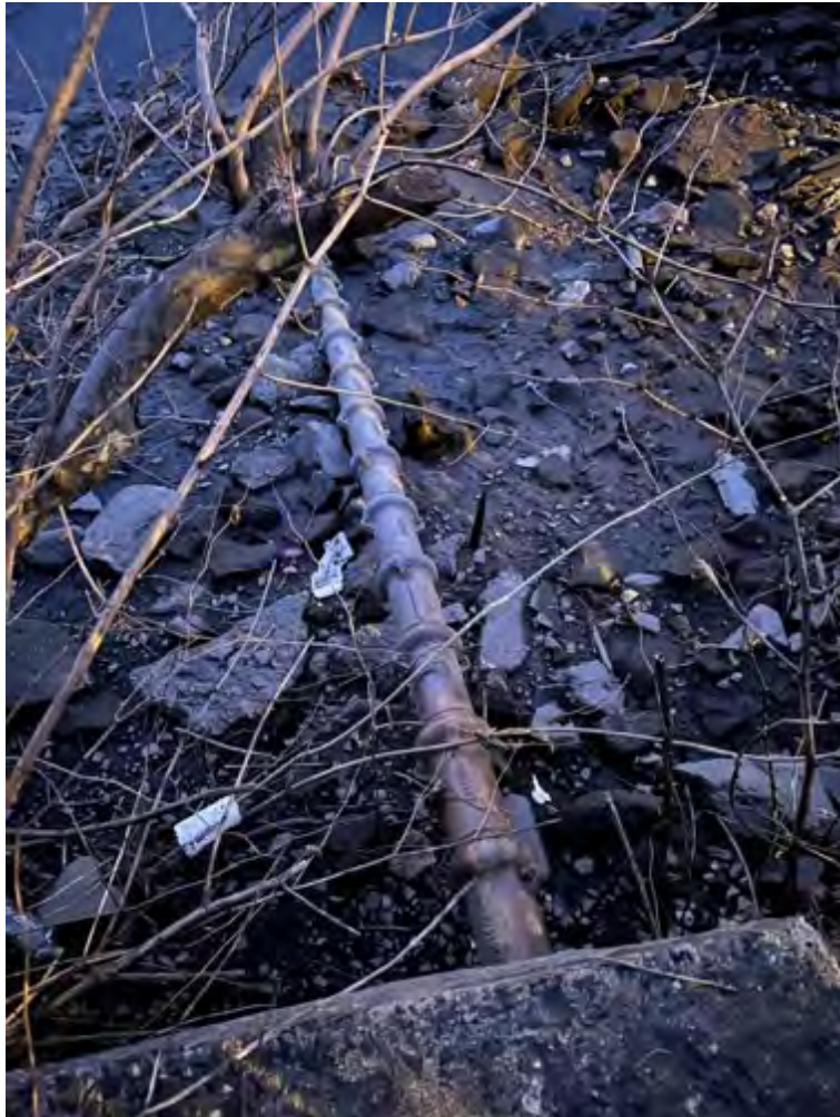
(A) Armored cable approximately fifteen feet from the water's edge. Passaic 3. January 2023, Belleville, New Jersey.
