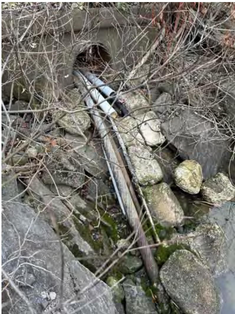
(D) Cables run under the road and into the Hudson River near the Mid-Hudson Bridge at Point of Interest: Hudson 3.1. January 2023. Highland, New York.
