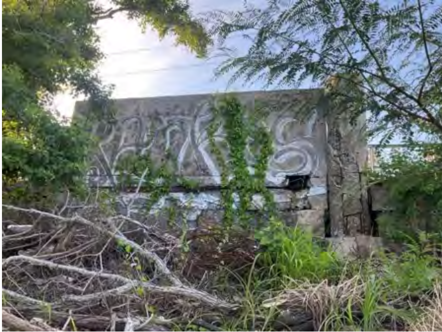
(K) New Orleans, LA. MISS 3.1. The small rectangle on the left is the passthrough for utility cables. June 2022.
