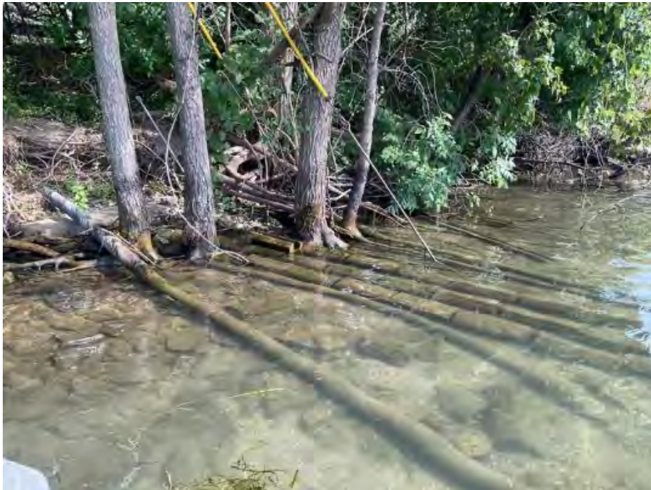
(C) Seven lead sheathed cables in the Detroit River. DR 1. July 2022, Trenton, MI.
