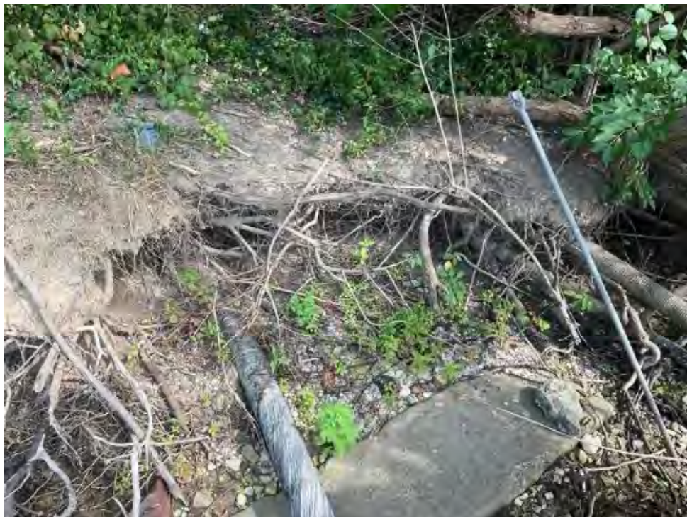
(D) Lead sheathed cables from (C) continuing past the tree line. They are buried in the ground and run up the hill to a Bell Systems manhole. DR 1. July 2022, Trenton, MI.
