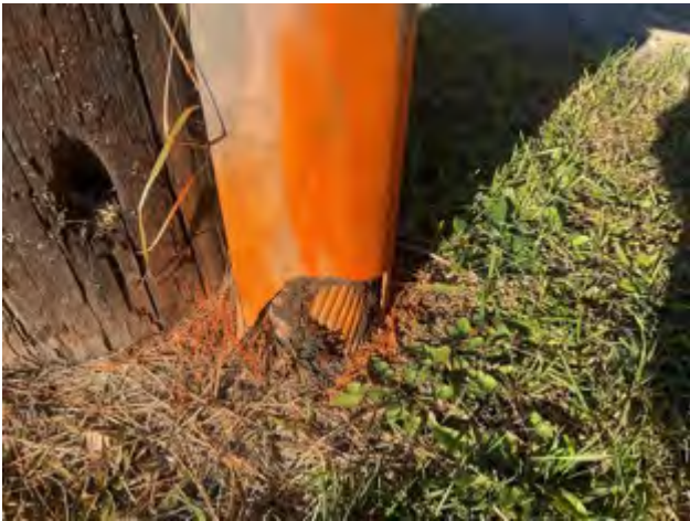
(B) Base of telephone pole in (A) and (C) showing marked cable going into the ground. October 2022. Natrona, Pennsylvania.
