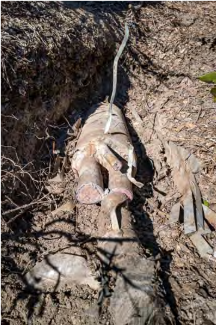
(A) Severed lead sheathed cables, and lead splice box on land. This photo was during a site visit with AT&T in January 2021.
