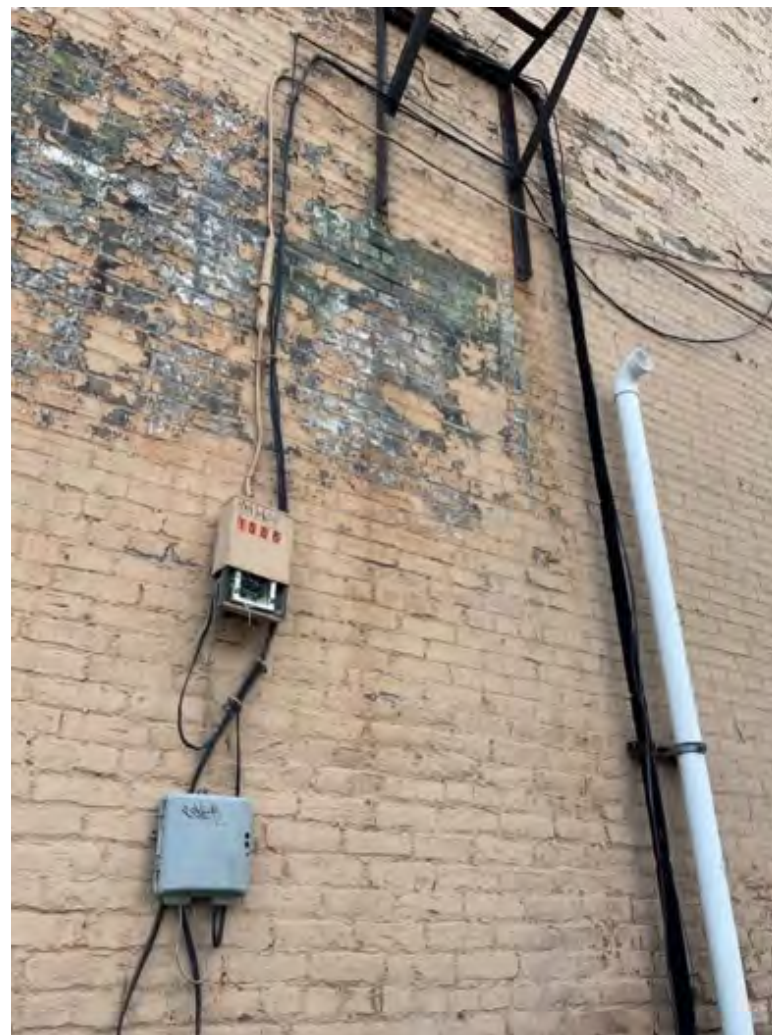
(B) End of the lead sheathed test line shown in (A). LH 2.3. July 2022, Bay City, MI.
