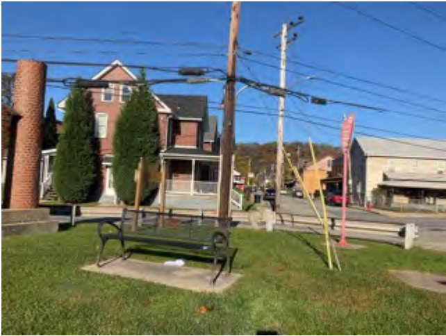
(A) Park bench near exposed lead sheathed cables and splice boxes. October 2022. Natrona, Pennsylvania.
