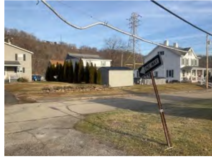
(F) CT11. Overhead lead sheathed cable running through a residential area near the end of town. February 2023. Coal Center, Pennsylvania.
