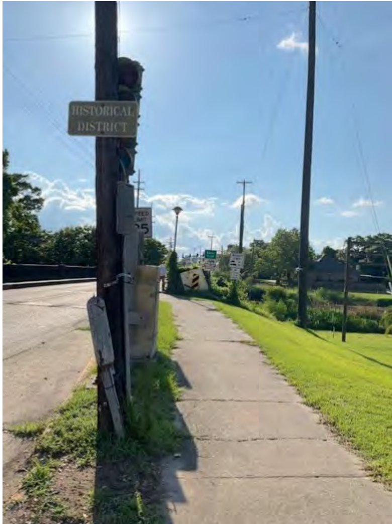
(G) Bare lead sheathed cables going into a lead splice box near the sidewalk leading into the Historical District. BT 24.1. June 2022, St Martinville, Louisiana.
