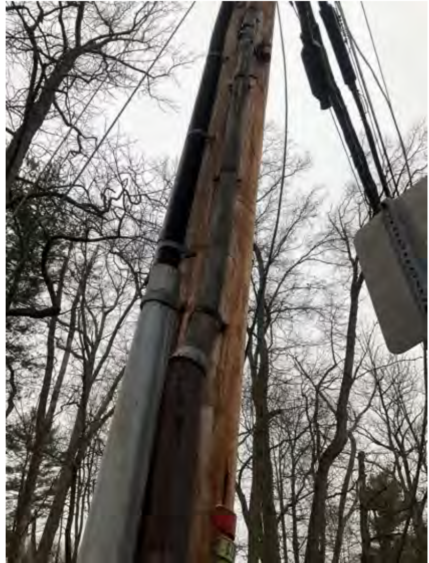
(J) Bare lead sheathed cable running up telephone pole in the Palisades. January 2023, Palisades, New York.
