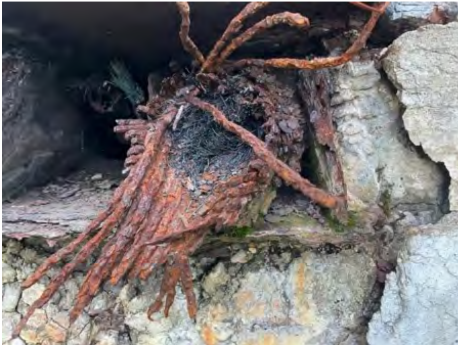
(J) New Orleans, LA. MISS 3.1. is an abandoned collection of cables.
