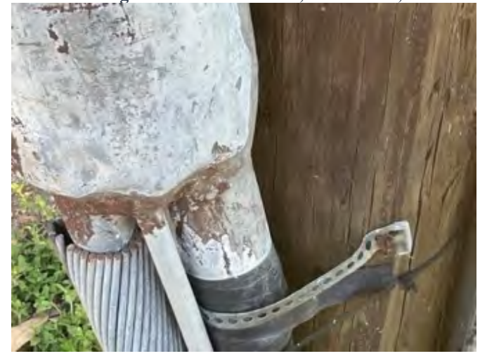
(F) Up close photo of bare lead sheathed cables coming from the bottom of a lead splice box (upper left corner of photo). BT 24.1. June 2022, St. Martinville, Louisiana.
