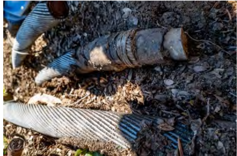
(B) Another splice location from land during the same site visit with AT&T in January 2021.
