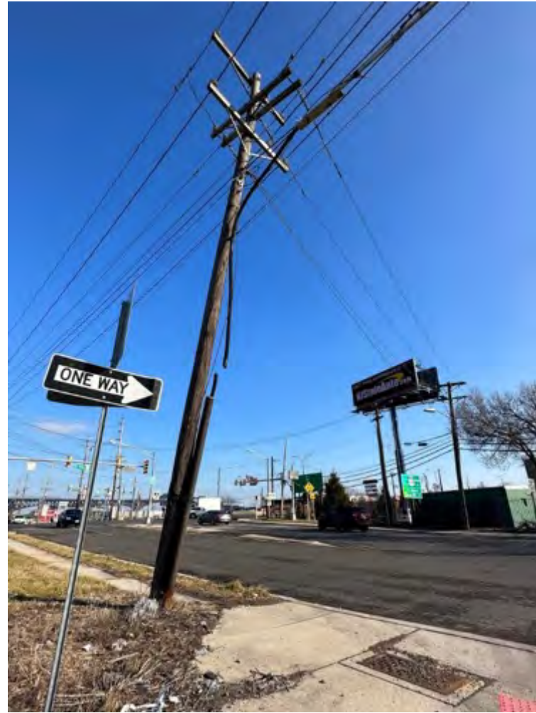
(B) Overhead cut, lead sheathed cables in the South Kearny area. There are two cables that run approximately 0.4 miles. South Kearny End A. January 2023, Kearny, New Jersey.
