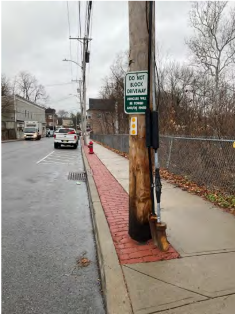
(K) Damaged lead sheathed cable at the base of a telephone in Wappingers Falls. Point of Interest: Wappingers Falls 3. January 2023, Wappingers Falls, New York.
