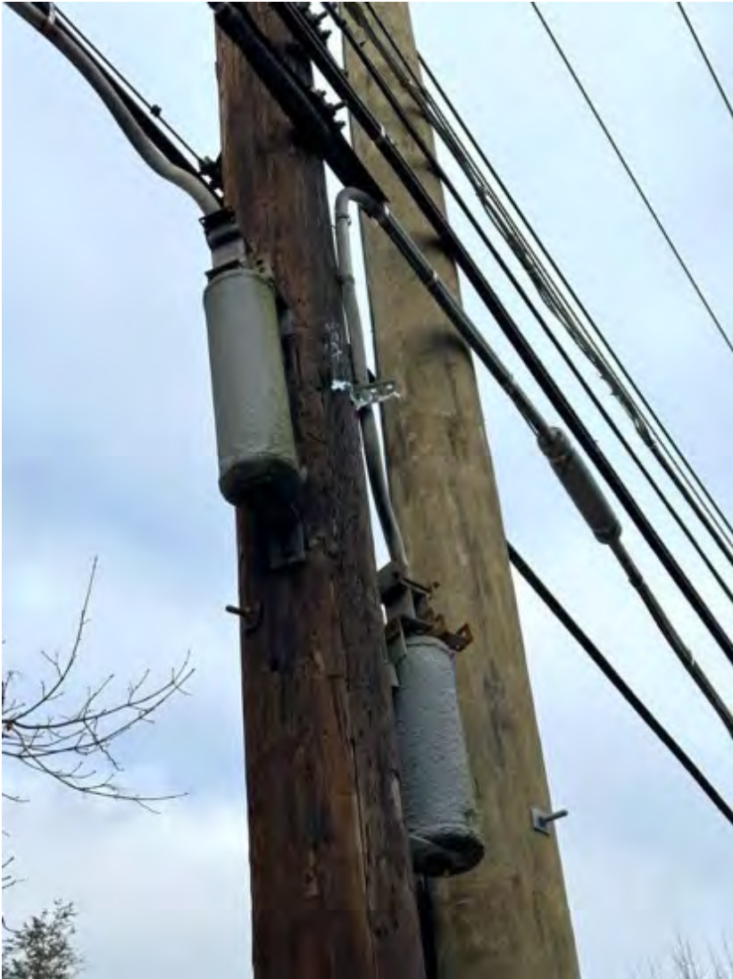
(A) Close up of telephone poles with overhead lead sheathed cable and leaded splice boxes. January 2023. Highland Falls, New York.
