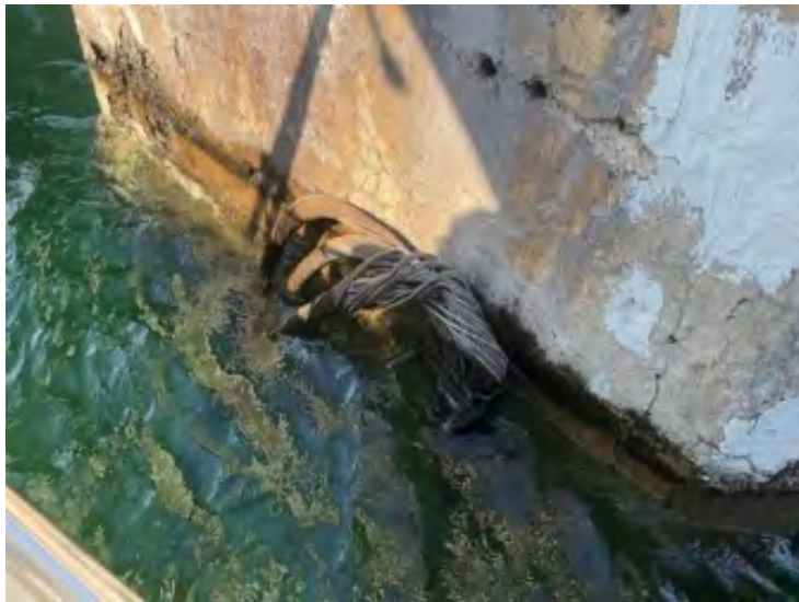
(C) Lead sheathed cables cut and hanging from bridge. Site LP 4.1. August 2022, Lake Pend Oreille, ID.
