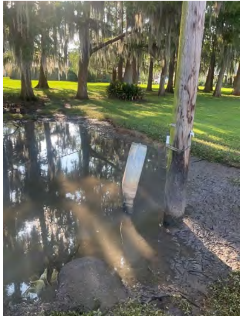
(H) Exposed lead splice box with attached cables and drainage into the Bayou Teche. BT 26.2. June 2022, Franklin, Louisiana.
