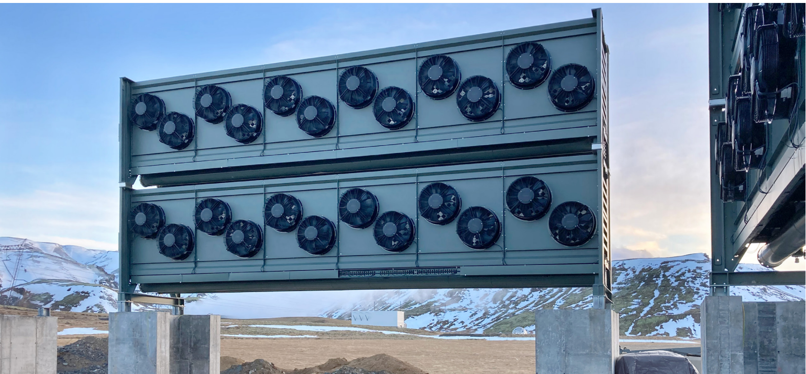
Climeworks direct air capture and storage plant in Iceland. Photo credit: Climeworks
