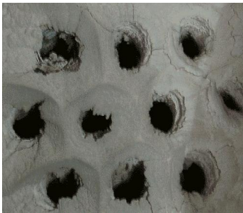
Dirty boiler tubes leading to decreased efficiency.
